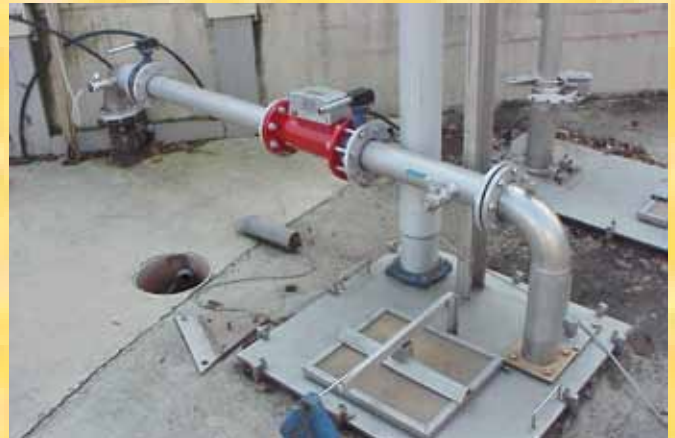
Biogas Flow Meter (Photo: P. Enzinger)
